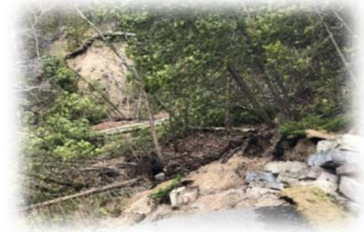
Little Traverse Wheelway Landslide, April 2020
