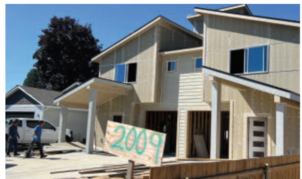
A multifamily home under construction under the BOCA (Building Opportunity and Choices for All) interim ordinance. Courtesy of the City of Spokane.
